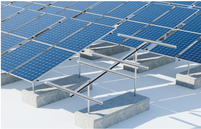
Magnelis Structure for Photovoltaic Panels Concrete Structure
