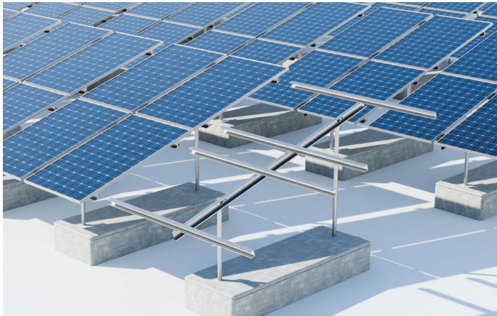
Magnelis Structure for Photovoltaic Panels Concrete Structure
